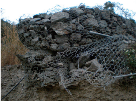
(a) 箱籠擋土工法破壞案例 1 (a) Box gabion retaining walls failure case No.1
