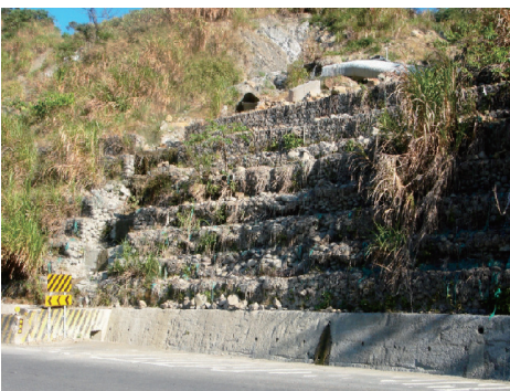
(e) 箱籠擋土牆破壞案例 5 (e) Box gabion slope protection failure case No.5
