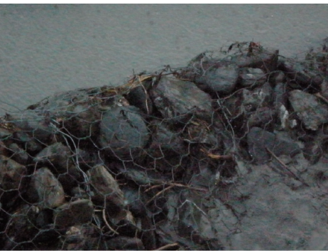
(c) 蛇籠護岸工程破壞案例 3 (c) Roll gabion bank failure case No.3
