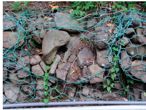
(b) 箱籠擋土工法破壞案例 2 (b) Box gabion retaining walls failure case No.2
